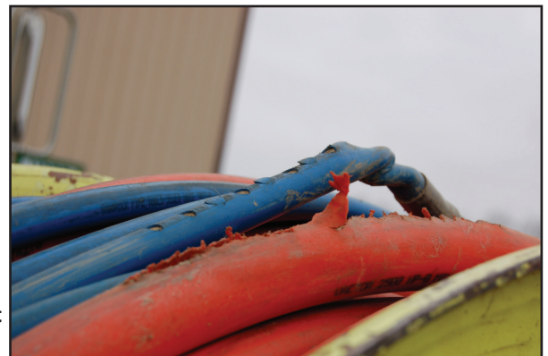
Right: An example of a hoses that should be immediately replaced.
